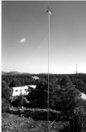
A Southwest Windpower Air 303, 300-watt turbine is the sole source of electricity for this remote home in northern Arizona.
